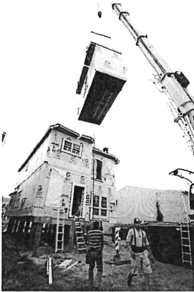
A crane places a section of a modular home being built to replace one destroyed by Hurricane Sandy in Manasquan.
